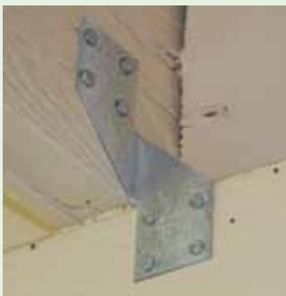
Figure 4-27. This is an example of retrofitting an existing house, originally built without hurricane clips. The popular H3 clip is used here; four nails attach the clip to the roof (truss-rafter) and four more nails attach to the wall or top plate below. For a retrofit, the clips are exposed on the outside of the house; therefore, both the clip and fasteners should be corrosion resistant and painted to blend with the exterior of the house. With the correct clip and nails you could perform the work or, if you prefer, hire a licensed contractor.
