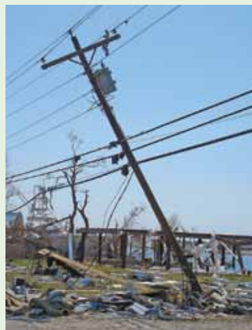
Figure 4-25. Downed or damaged power lines in a residential area can pose a serious danger to public safety. Source: U.S. EPA
