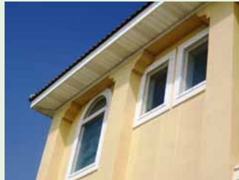
Figure 4-17. Flat impact polycarbonate panels are installed directly over windows of a coastal home. This window covering provides excellent storm protection with minimal aesthetic impact. Source: Roll-a-way/QMI
