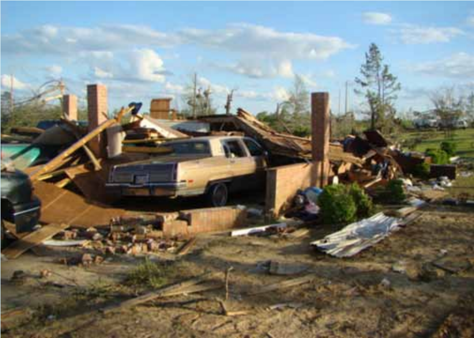
Figure 2-1. Major tornado damage in Yazoo County, MS, in April 2010. Source: NOAA National Weather Service, Jackson, MS.
