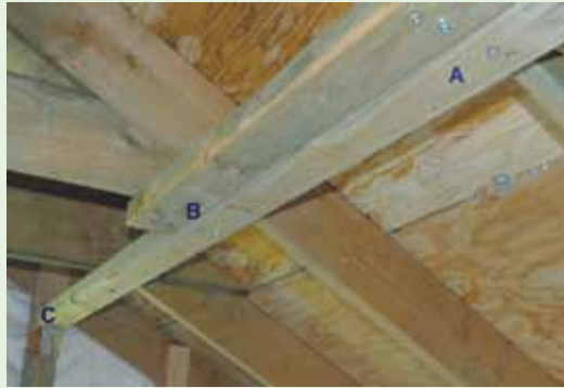
Figure 4-3. In this application of lateral bracing, the 2 x 4's are 18 inches from the ridge and connect to horizontal members that attach the opposing trusses. Not all roofs will have the horizontal members. The 2 x 4's are connected with two #14 3-inch screws (A) and overlap over two trusses (A and B). The end is connected to the gable end with an angle or L bracket (C).
