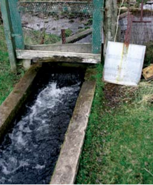
2.2 Water being diverted from a stream into flow-through raceways for trout production. Chris Hartleb
