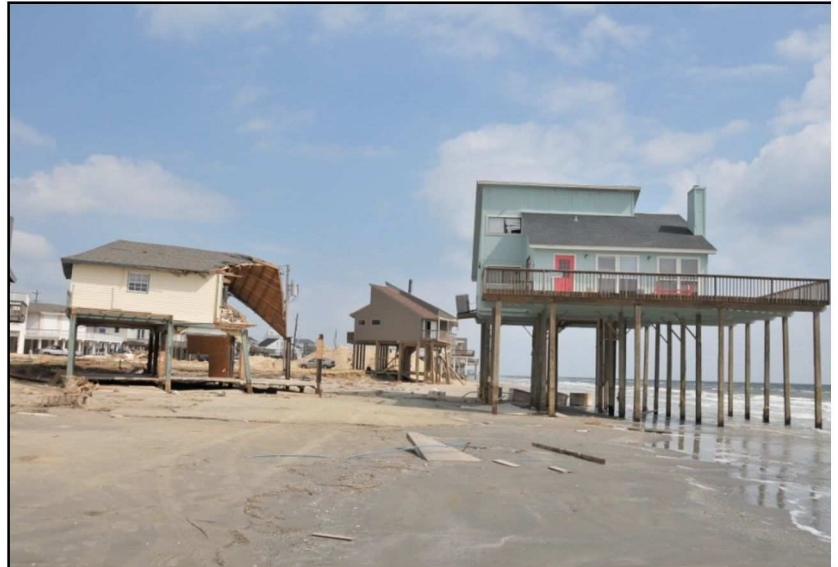
Figure 3 – Galveston Island, Texas after Hurricane Ike – October 2008. The house on the right is built to V-zone standards but has migrated into the waterline. The house on the left was also elevated, but not sufficiently high and was damaged. Texas has no shoreline setback.
