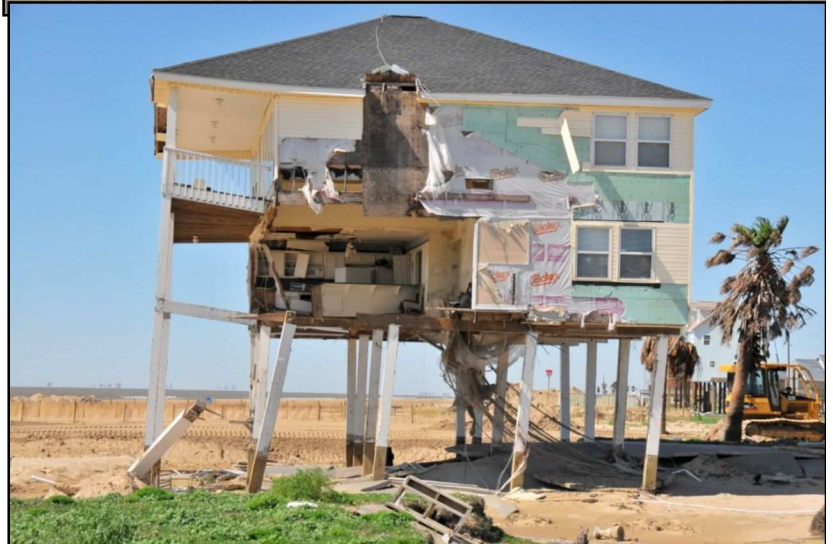
Figure 4 – Bolivar Peninsula, Texas – March, 2009 – Damage to structure after Hurricane Ike. Although the structure was heavily engineered for wave action, it was too close to the shore. The storm surge exceeded design levels damaging the house. The structure is now encroaching on the beach. Migration is evidenced by the erosion and scour as shown by uncovering of the unpainted portion of the support columns.
