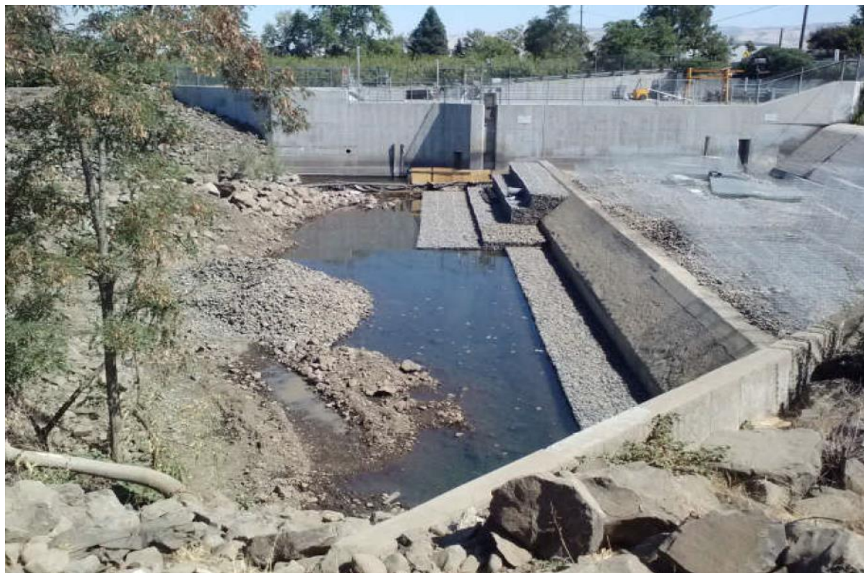
Figure 5. Corps of Engineers repairs to the Nursery Bridge Spillway in 2014, to address stability concerns.
