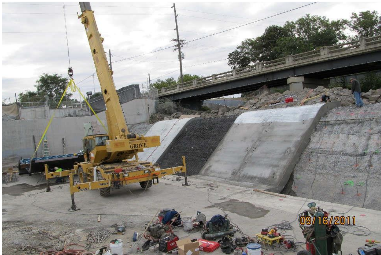
Figure 4. Replacement of degraded concrete on the Nursery Bridge Drop Structure Spillway in 2011 (Photograph provided by John Wells).
