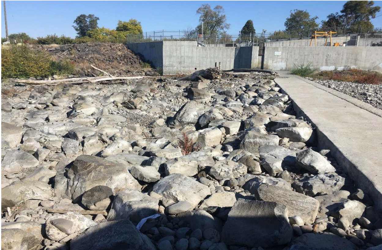
Figure 6. Roughened riffle installed by the Corps of Engineers below the Nursery Bridge Drop Structure in 2017.
