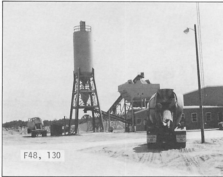
Figure 48. A site for the preparation of ready-mixed concrete at Nags Head. The vicinity is undergoing much construction and this plant provides concrete for building sites.
