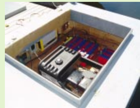
Generator and battery bank for powering floating upweller systems in remote locations. Photo by Robert Rheault.
