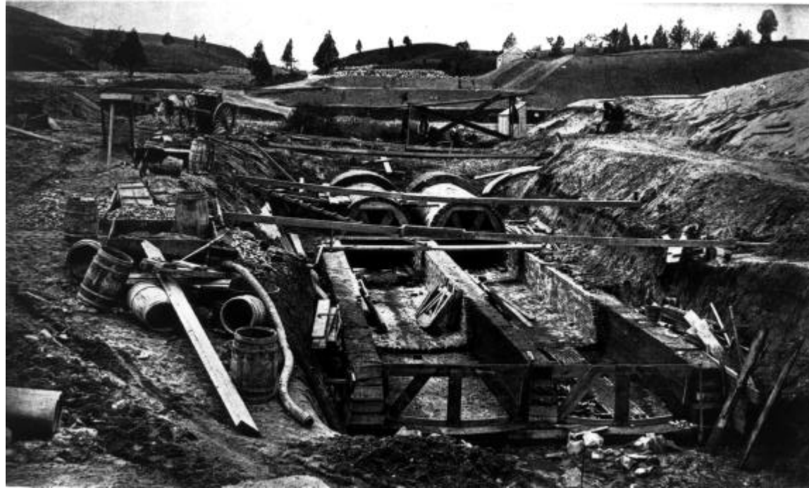
Plate 9 Construction of sewers at Field's Point. From the 1891 Annual Report of the Providence City Engineer.
