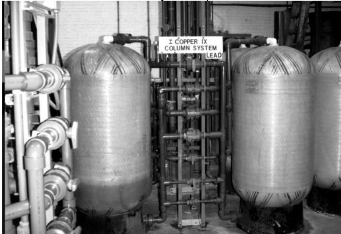
Ion exchange cylinders – part of the modern pretreatment system for removing copper and lead from wastewater at Victory Finishing Technologies, an electroplating facility in Providence, R.I.
