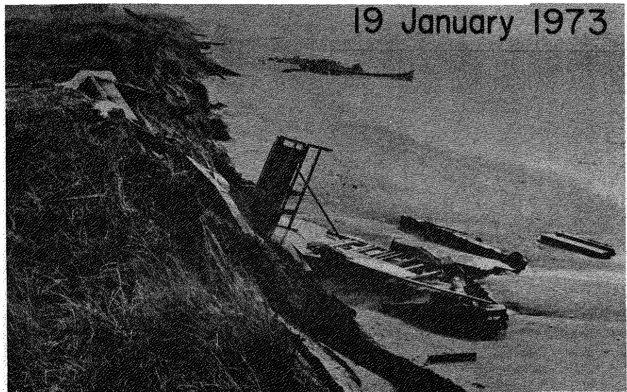
Fig. 2. Erosion and destruction of the house under construction on lot 226 of Siletz spit.
