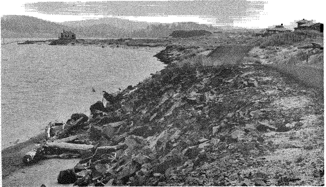
Fig. 14. Riprap placed on the bay side of the spit to prevent or decrease erosion.
