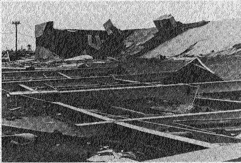
Fig. 2. The remains of a building after the walls were collapsed by winds of Hurricane Celia. Photo by Texas Highway Department.
