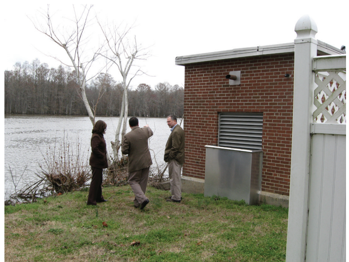
Pumping station adjacent to Roanoke River
