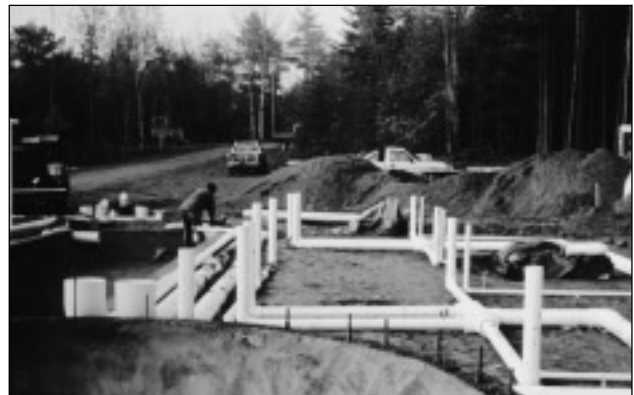
Figure 3. This shows the sump for a swirl-separator at a lobster transshipment facility we built in Boothbay, Maine. A swirl separator is a centrifugal filter that operates passively. The pipes are the manifold distribution–water supply lines to the area where the bio towers are going to be.
