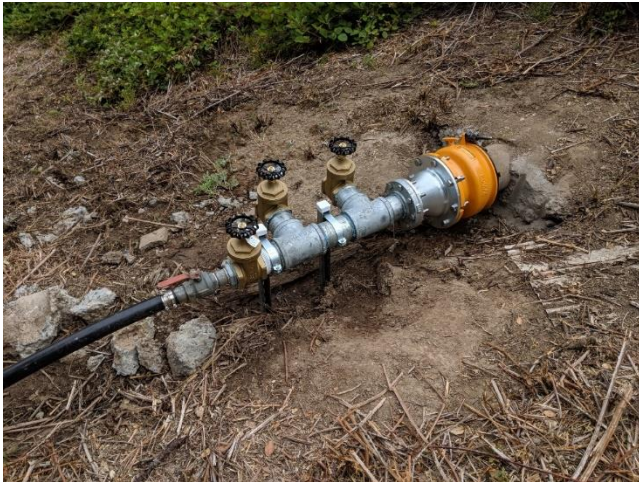
Figure 62. Improved pond outlet manifold for the GVF release, photo courtesy of GRRCD, July 2019.
