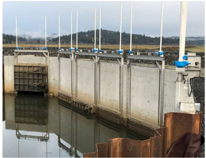
Winter Lakes tide gate project. (photo courtesy of Beaver Slough Drainage District)
