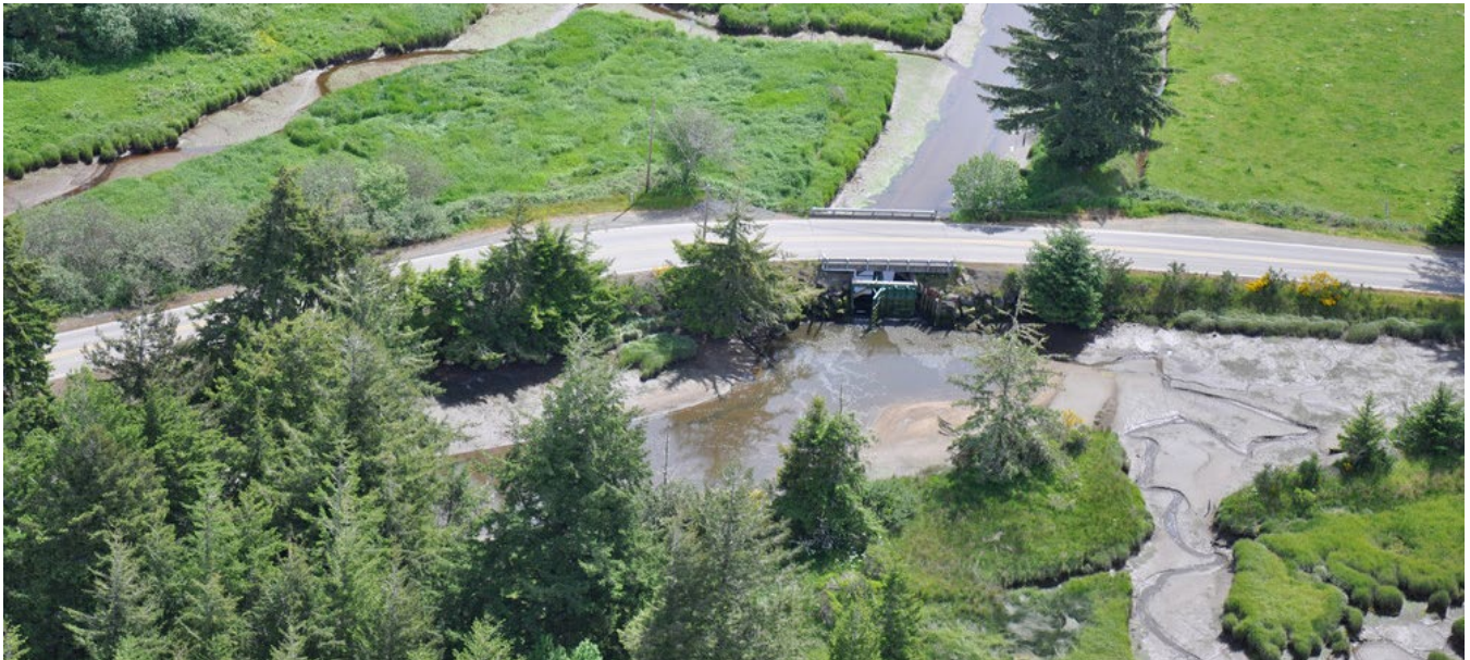
A road crosses over a tide gate at Willanch Creek. (photo courtesy of Oregon ShoreZone, CC-BY-SA)
