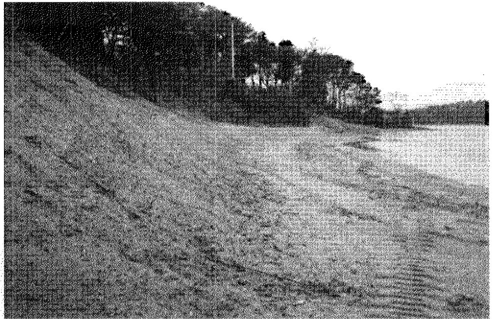
Fig 35. Fiber rolls covered with sediment
