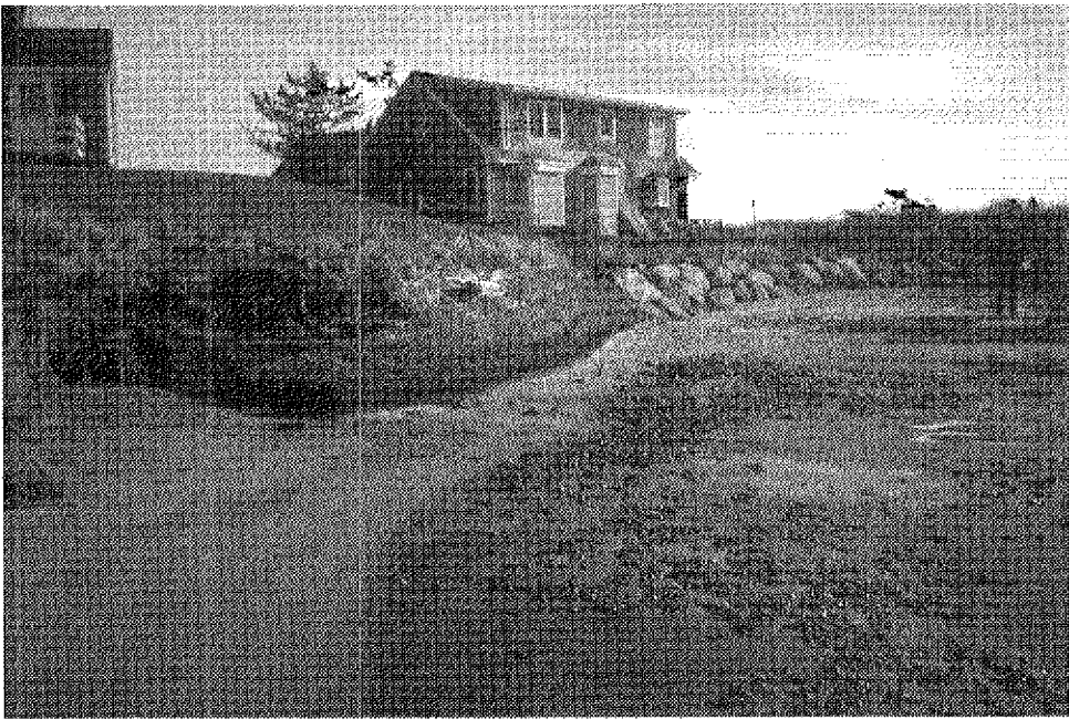
Fig 6. End scour on flanking erosion around bio-logs
