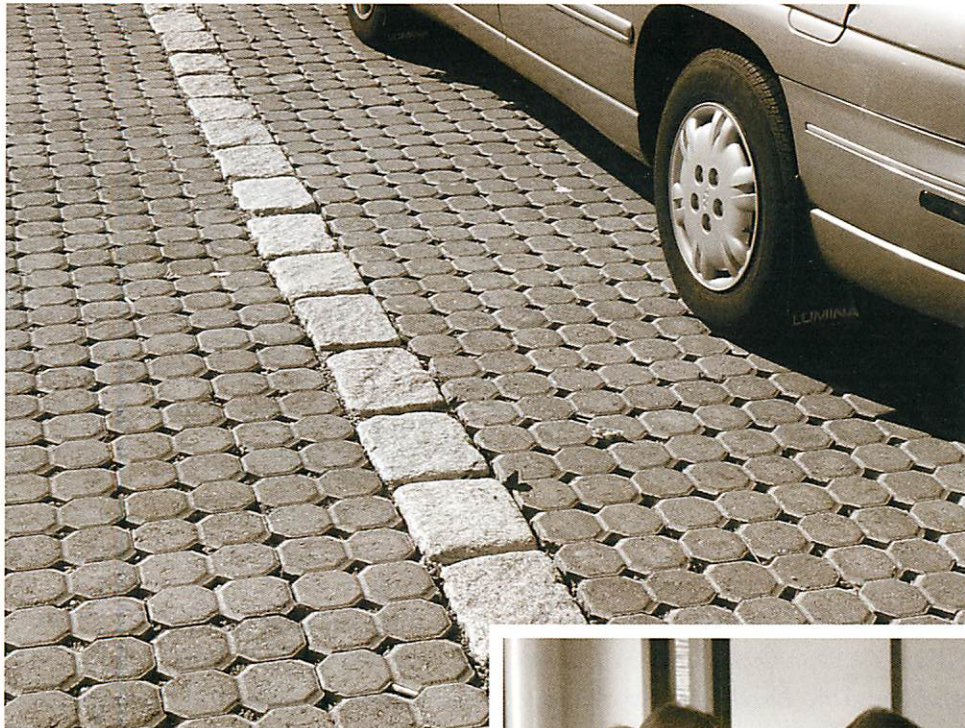
Public access parking stalls at Cornfield Point, Old Saybrook feature alternative pavement that promotes infiltration. Shown here are modular concrete pavers.
