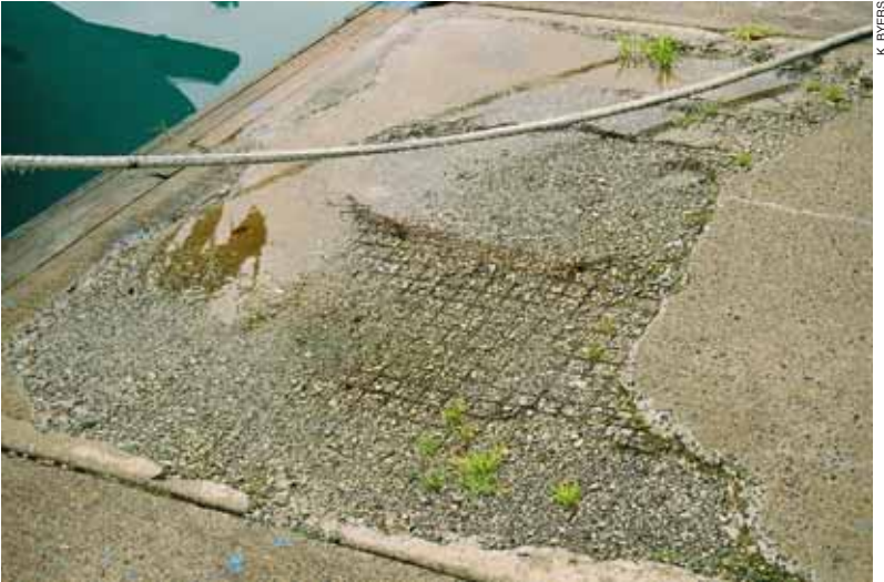
Degradation of concrete float, showing exposed reinforcing steel, grass growth, and standing water.
