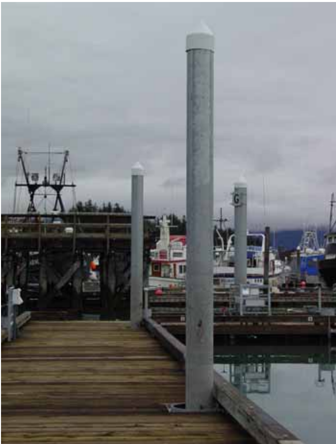
Round steel piles, aligned in piling guides. The guide structure needs to accommodate loads imposed by the dock, wind, current, and moored vessels.
