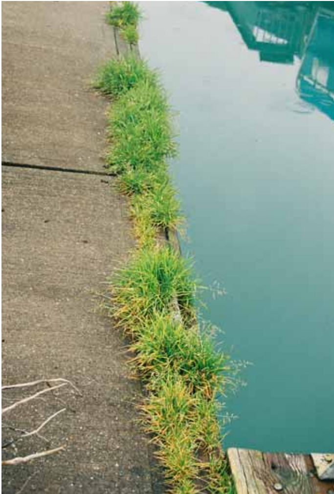
The growth of grass between concrete and wood indicate excessive moisture.
