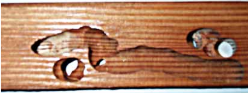
Shipworm damage to a section of a Southeast Alaska vessel hull. Tunnels are \frac{1}{2} inch in diameter.
