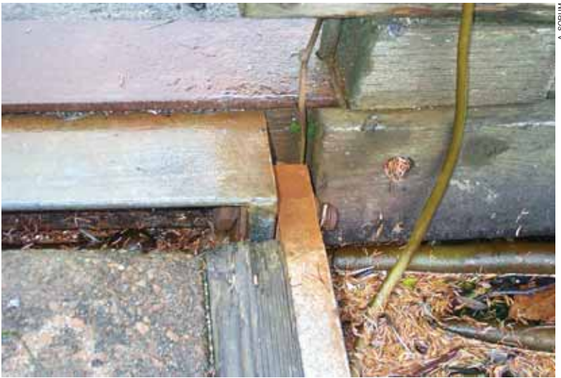
Failed dock-to-dock connection.
