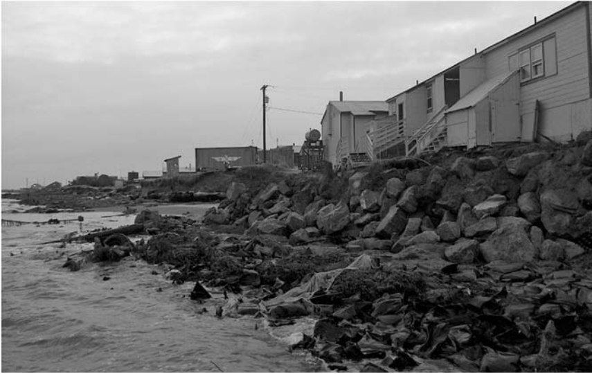
Figure 2. In Shishmaref, Alaska, engineering “solutions” have been ineffective.
