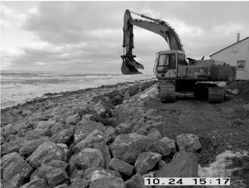
Figure 1. Shishmaref emergency bank protection. Top photo October 2004, bottom photo October 2005.
