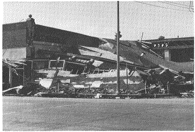
Fig. 20. After the masonry wall in Corpus Christi yielded to the winds of Hurricane Celia (1970), the roof fell. Photo courtesy of the Texas Highway Department.
