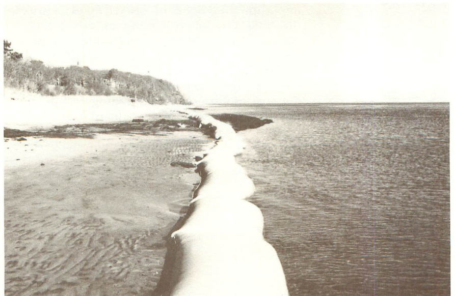
Experimental coastal erosion control project uses sill bag method to raise beach.
