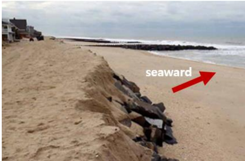
Figure 1.1: Partially exposed relic rock seawall after Hurricane Sandy (Irish et al. 2013)
