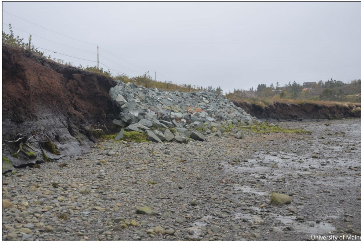
Figure 7. Rip-rap wall on the bluff at the north side of the Lubec Heath, October, 2014. Note that the heath embankment next to the nearby end of the riprap is farther landward than on the left side of the image. This suggests increased heath erosion and shoreline retreat from waves interacting with the wall.
