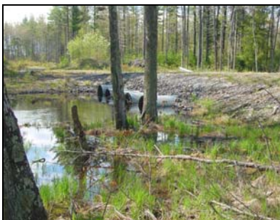
Figure 13. A second culvert downstream from W7, also with standing water.
