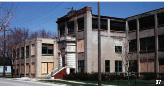
Before: Abandoned facility contaminated with heavy metals, petroleum and other organic chemicals from nearly 100 years of manufacturing use.
