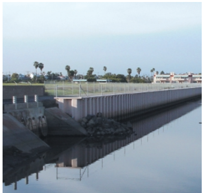
Talbert Channel D2 adjacent to the Banning Ave. Storm Water Pump Station
