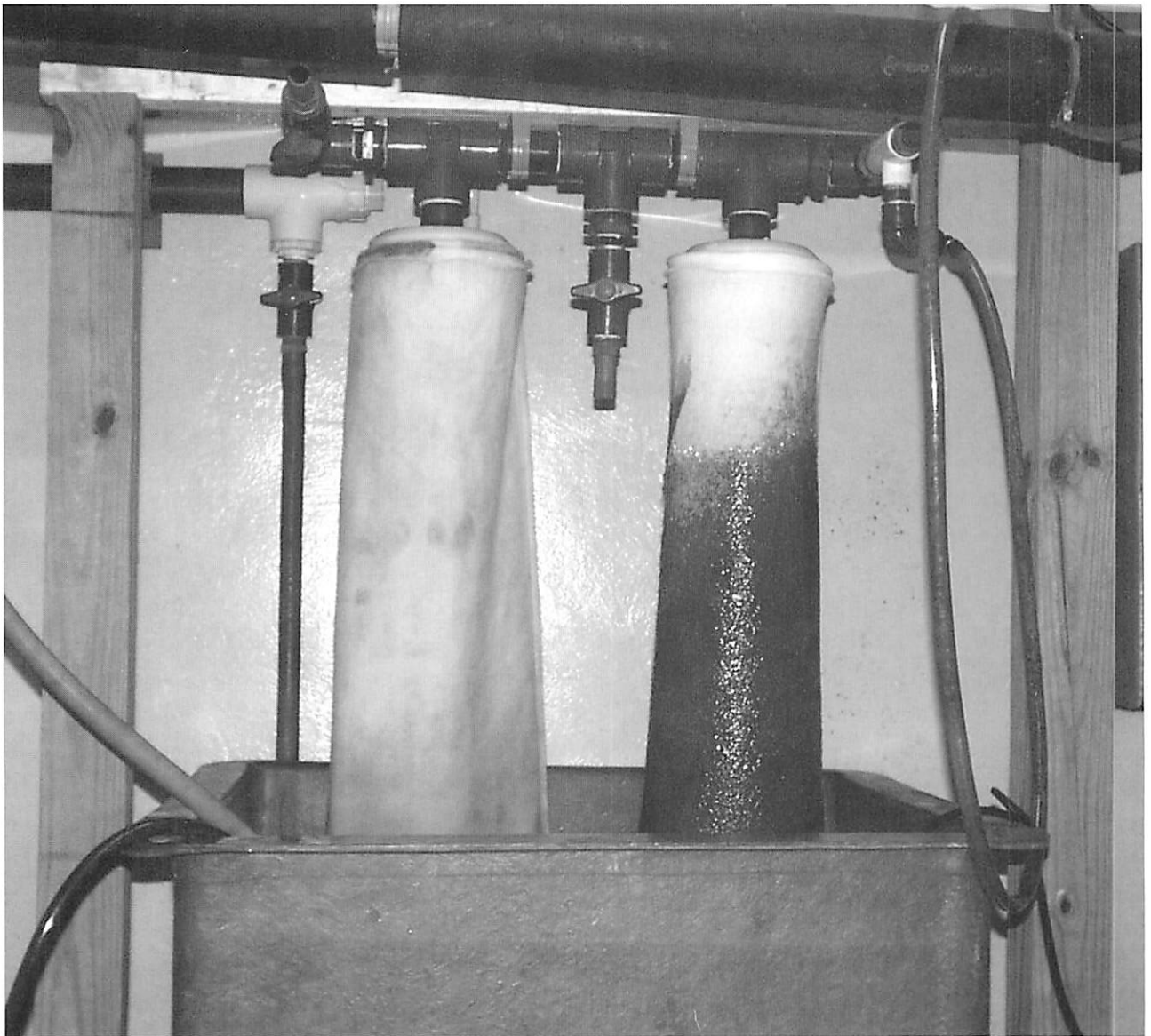
Figure 23. Bag filter systems for filtration of seawater.
