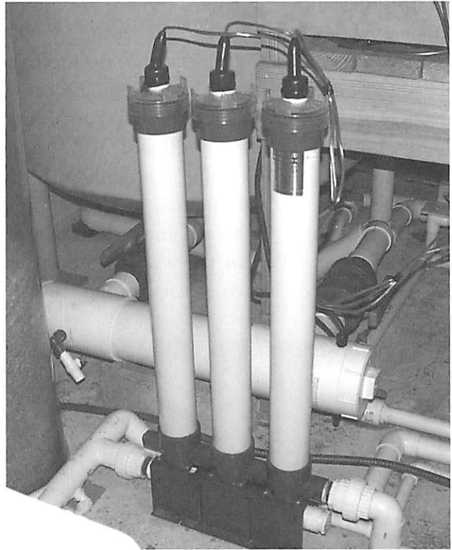
Figure 24. Ultraviolet (UV) light systems for sterilizing seawater.
