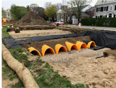
Longfellow Park Infiltration
