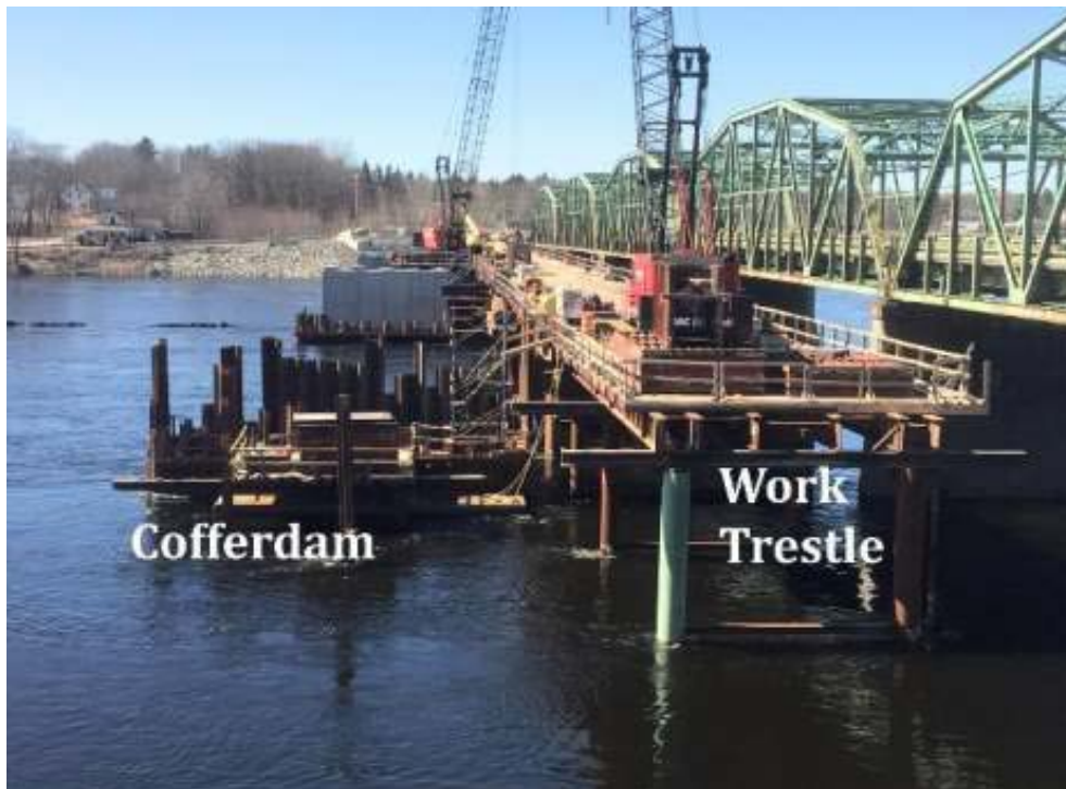
Figure 2: Example of a pile-supported temporary work trestle adjacent to a sheet pile cofferdam
