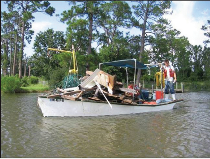
Figure 17: Debris removal, Back Bay Biloxi, Mississippi. Photo: NOAA
