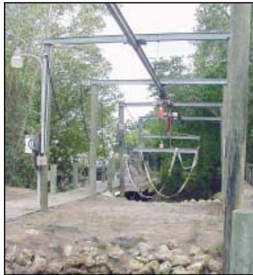
Boat lift at Flamingo Bay.
