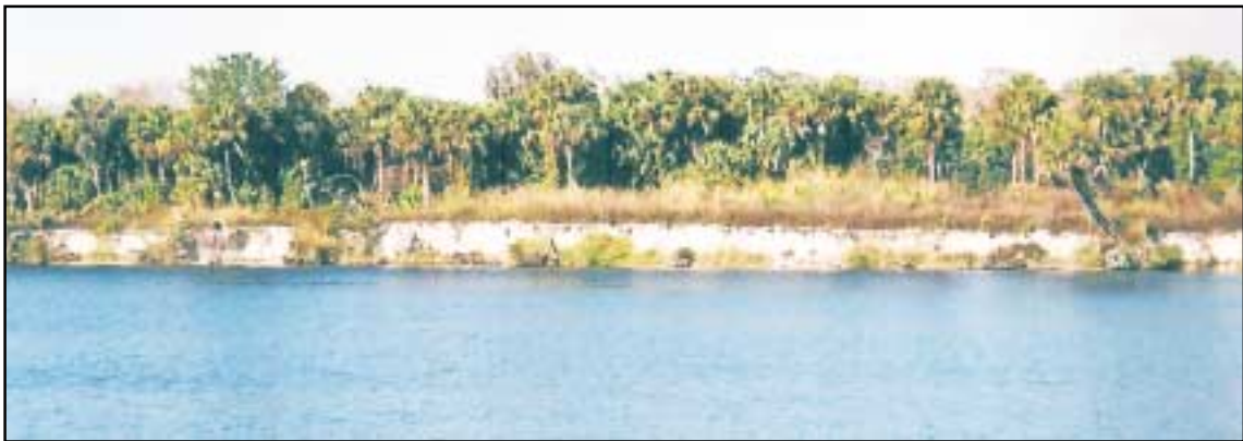
Figure 16. Side cast spoil along waterway at Rialto.
