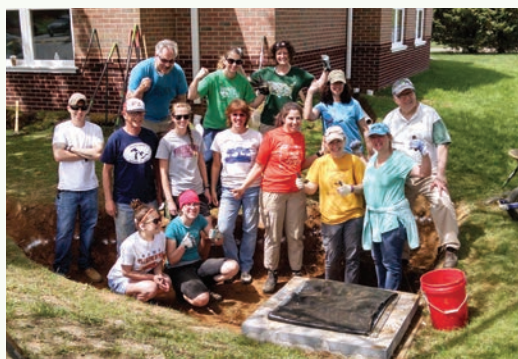
CECIL COUNTY WATERSHED STEWARDS ACADEMY participants take a break after completing the hard part of excavating a rain garden at the Rising Sun Public Library. PHOTO BY ERIC BUEHL
