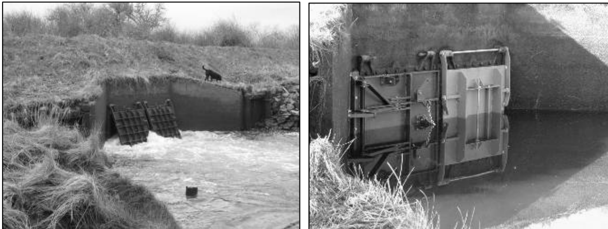
Figure 2. Tide gates at Vera Slough before (left, open) and after (right, closed) replacement with experimentally modified designs.
