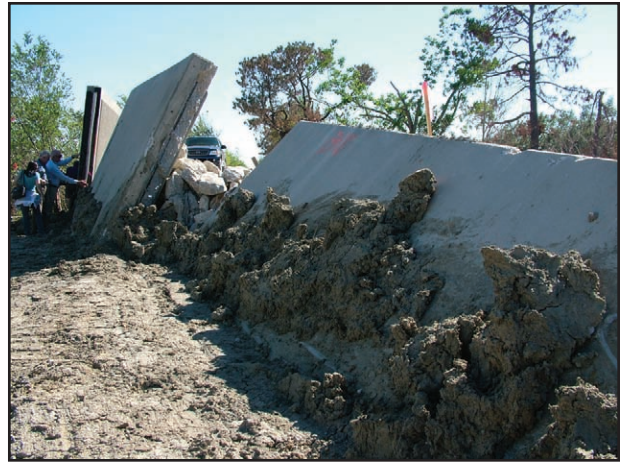
New Orleans' failed levees and floodwalls contributed to the severe storm damage suffered by many Louisiana Sea Grant constituents.
