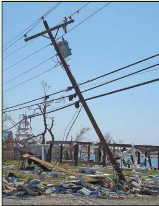
Figure 31. Downed or damaged power lines in a residential area can pose a serious danger to public safety. Source: EPA.
