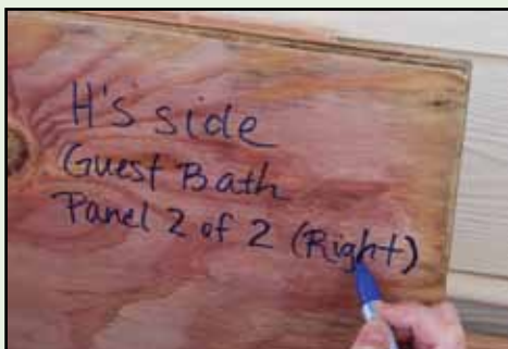
Figure 27. After the plywood is cut for each window, each piece should be labeled so the panels for one window are not mixed with those for another. It would also save time to indicate on the panels, well before any threat of a storm, where the fasteners will be attached.
