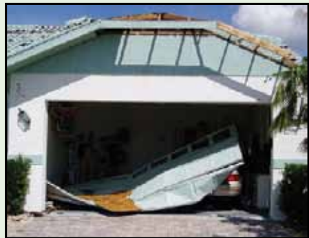
Figure 29. Because of their width, double-wide garage doors are more susceptible to wind damage than single doors. The wind can force it out of the roller track, especially if the track is lightweight or some of the anchor bolts are not in place. This occurs because the door deflects too much under excessive wind pressure and fails. You should reinforce your garage door by installing horizontal and/or vertical bracing onto each panel, using wood or light gauge metal girds bolted to the door mullions. You may also need heavier hinges and stronger end and vertical supports for your door. Source: Florida Hurricane Depot.
