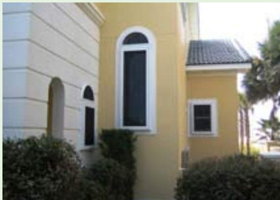
Figure 4-16. In-place stainless steel impact screen protects several windows of a coastal residence. This system requires no deployment and provides shade. Source: Roll-a-way/QMI
