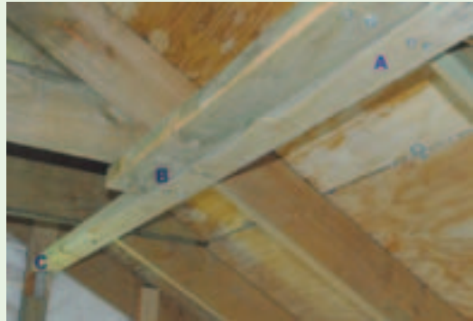
Figure 4-3. In this application of lateral bracing, the 2 x 4's are 18 inches from the ridge and connect to horizontal members that attach the opposing trusses. Not all roofs will have the horizontal members. The 2 x 4's are connected with two #14 3-inch screws (A) and overlap over two trusses (A and B). The end is connected to the gable end with an angle or L bracket (C).
