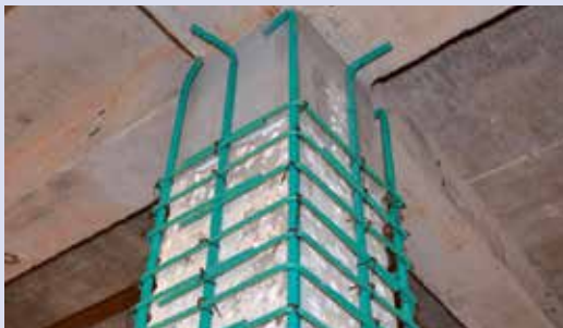
Figure 4-47. Example of epoxy coated rebar about to be encased in concrete. Any bends or cuts in the rebar that cause the epoxy to come off should be recoated.
