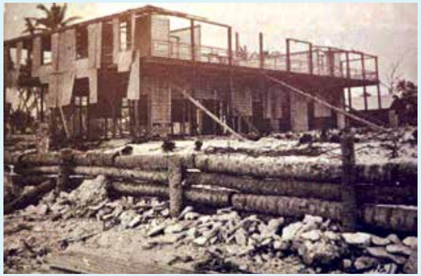
Figure 2-6. Typhoon Wind Impacts - Damage to the Catholic Girl's and Nuns' Living Quarters building in Jaluit after the 1905 typhoon. Note the blown off roof, which is common from the strong winds of a typhoon. In addition, there is water damage or inundation that overtopped the log seawall and eroded or scoured sediment behind the wall (Photo Micronesia Area Research Center).
