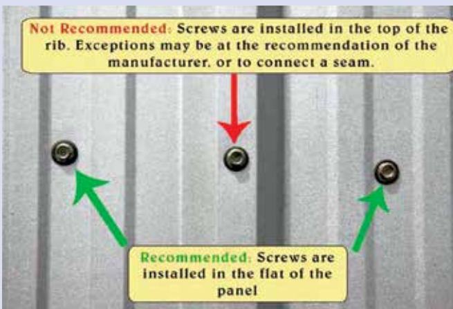
Figure 4-24. Some roofs in Majuro have flat sections that differ from undulating roof sheets shown in Figures 4-20 and 4-23. In this case, fasteners to the purlins should be in the flat lower flat portion of the panel. Photo courtesy of Christian Oakes, IOM.
