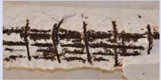
Figure 4-46. Rebar in direct contact with concrete with salt content can cause corrosion of the rebar. Thus, there may be a need to epoxy coat the rebar.
