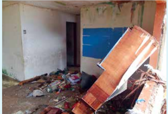
Figure 2-17. During the March 2014 event, about 110 homes were damaged and about 940 family members were displaced and sought sanctuary in government-designated shelters and churches. It is because of damage such as this that Part 4 of the handbook covers tools to reduce damage such as elevating of structures or building with flood resistant materials.
