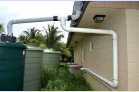
Figure 4-52. First-flush systems help to keep your water catchment system clean and reduce the need for maintenance. Dust, debris, or fecal matter that collects on your roof is washed off when it begins to rain and collects in the diversion pipe to the right. After a sufficient amount of rain has washed the roof, and the diversion pipe is full, either a pipe bend or a floating ball valve diverts water to the left where it is collected in the water tank.
