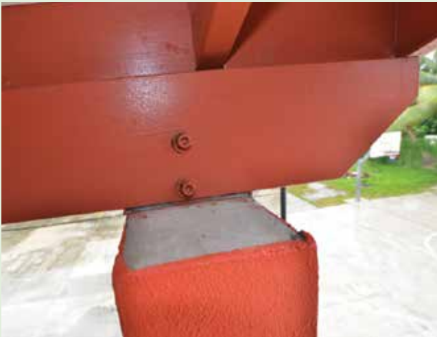
Figure 3-9. This roof truss is connected to the CMU column with a bolted plate to prevent roof uplift during strong winds. Connection of roof trusses to the walls, beams, or columns is also important for residential houses and is covered in Part 4.
