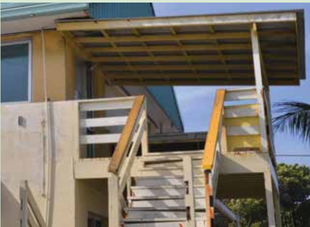
Figure 3-13. Some sturdy reinforced-concrete buildings have wood stairs to the second floor. They are likely to be damaged or washed away during heavy wave inundation. Such contingencies need to be planned for by having an emergency ladder readily accessible on the second floor. Note that the roof over this upper landing is also likely to be damaged or blown away during a typhoon. Photo of the Majuro Youth Center.
