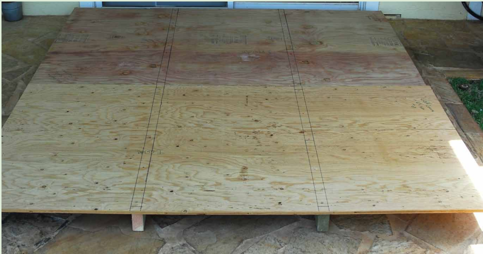
Figure 4-35. During assembly of the shutters in Figure 4-28, the two panels to be joined sit atop the 2 by 4's. The outline of the 2 by 4's and all screw locations are marked on the panel. Panels should be cut, labeled, and marked as to all fastening locations before hurricane season. The panels can be quickly attached with wood screws drilled from the plywood panel into the 2 by 4. The panel is then raised with the end near the window being the pivot point. The panel is then attached to the structural framing of the window as shown in Figure 4-34.
