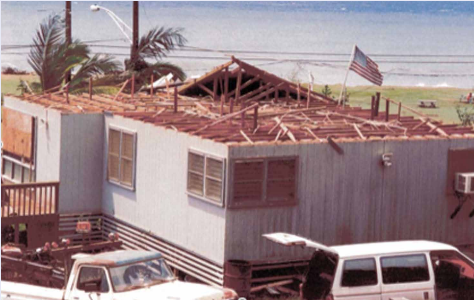
Figure 2-6. A common site on Kauai after Hurricane Iniki. Many roofs were blown off due to a lack of proper connection. Photo courtesy of Department of Commerce and Consumer Affairs Insurance Division.
