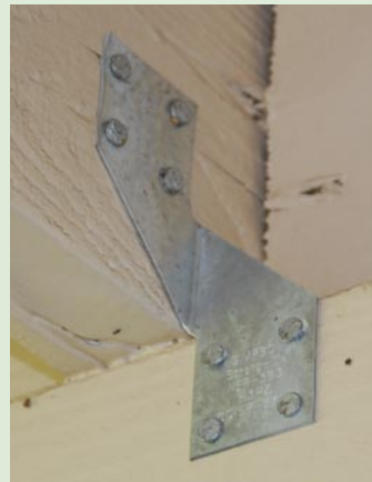
Figure 4-4. This is an example of retrofitting an existing house, originally built without hurricane clips. The popular H3 clip is used here; four nails attach the clip to the roof (truss-rafter) and four more nails attach to the wall or top plate below. For a retrofit, the clips are exposed on the outside of the house; therefore, both the clip and fasteners should be corrosion resistant and painted to blend with the exterior of the house. With the correct clip and nails you could perform the work or, if you prefer, hire a licensed contractor. 20
