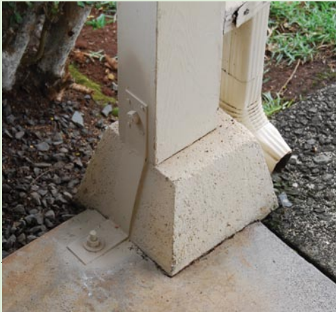
Figure 4-6. In some retrofit examples, it is possible to tie a portion of the house to the foundation. Here, a metal strap connects the vertical post to the foundation, which finishes the continuous load path connection from roof to the foundation. Photo courtesy of Hurricane Protection Services.
