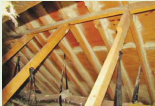
Figure 4-5. Spray polyurethane foam is used to add strength between the rafters and the plywood sheathing. This method can be used to strengthen existing roofs and may negate the need to replace older roofs. It can also be used where fasteners are missing or at the corners of hip style roofs or the ends of gable end roofs, which are especially susceptible to wind forces. See FEMA publication numbers P-499 and P-804. Image courtesy of FEMA
