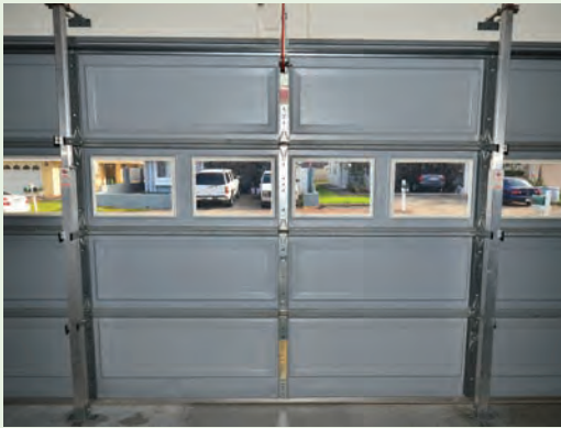
Figure 4-23. Vertical braces such as these can be deployed during high-wind events to strengthen the garage door. The braces are secured from the header over the garage door to the fasteners installed in the concrete floor. Deployment and breakdown are about 10 minutes each. The windows have been covered with a laminate film. Image courtesy of Dennis Hwang
