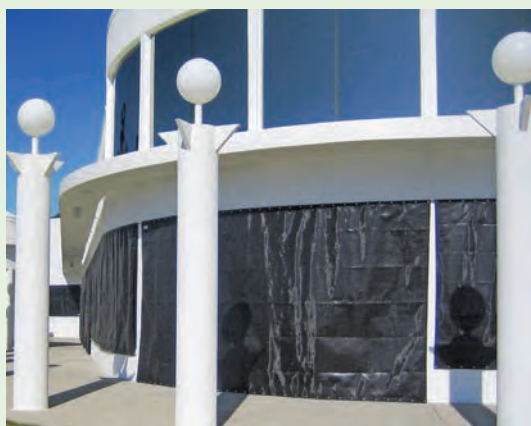
Figure 4-17. Polyethylene basketweave fabric windscreens deployed directly over ground floor windows of a coastal home. Image courtesy of Roll-a-way
