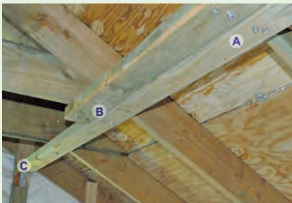
Figure 4-3. In this application of lateral bracing, the 2"x4"s are 18 inches from the ridge and connect to horizontal members that attach the opposing trusses. Not all roofs will have the horizontal members. The 2"x4"s are connected with two #14 3-inch screws (A) and overlap over two trusses (A and B). The end is connected to the gable end with an angle or L bracket (C). Image courtesy of Dennis Hwang
