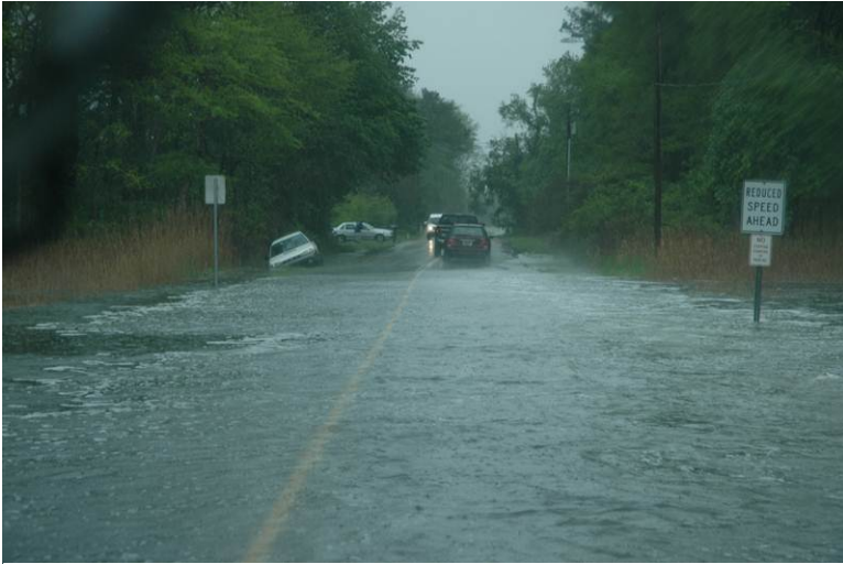
Figure 3.1: Flooded roadway (New Road) during 2008 northeaster.
