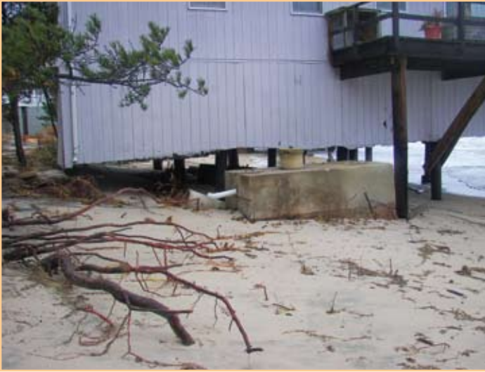
Damaged or cracked tanks and broken pipes can be flooded, allowing septic waste to escape into adjacent waterways and properties.
