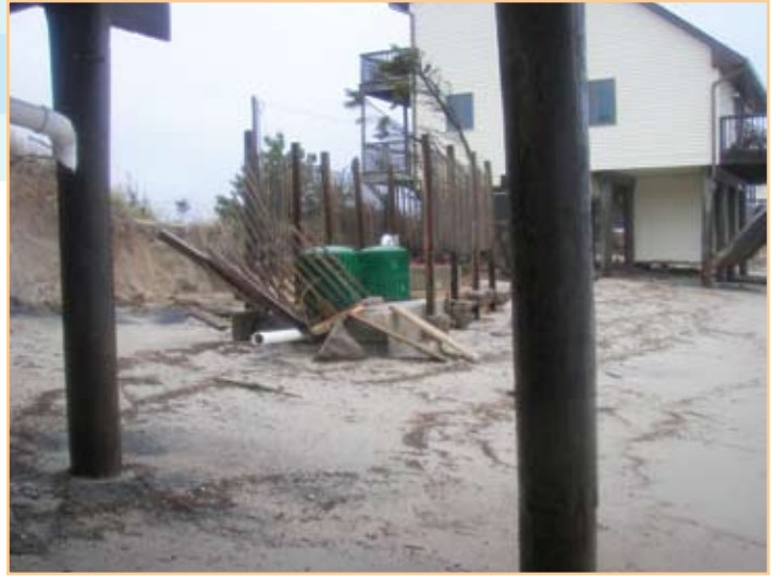
When a tank is exposed, the sewer line from the home is usually severed, making the house uninhabitable.
