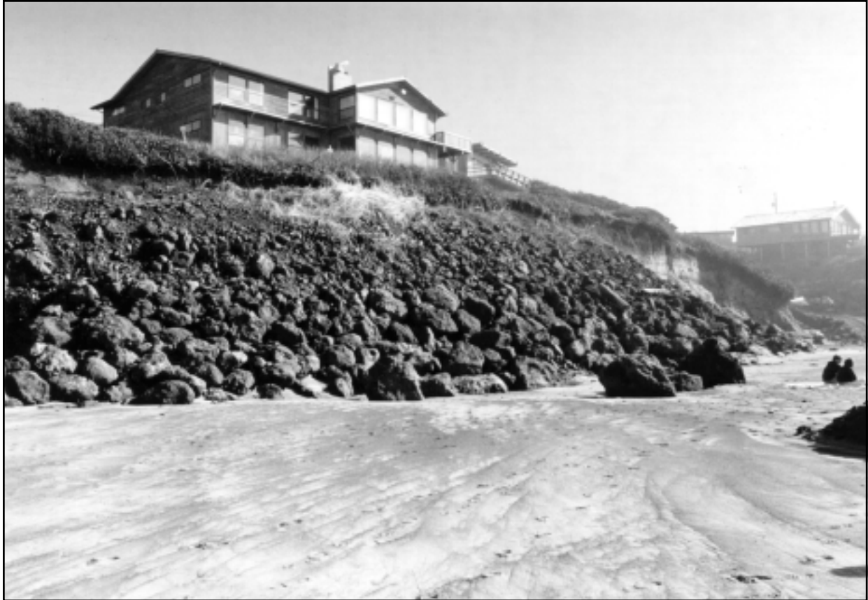
Riprap revetments often extend out onto the public beach, as illustrated here at Gleneden Beach (J. Good photo).
