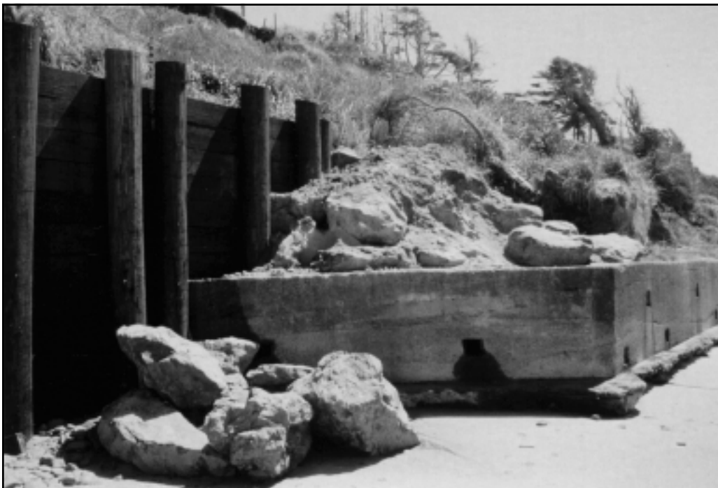
A new timber-pile retaining wall (left) and old concrete-reinforced seawall (right) at Arch Cape on the northern Oregon coast (J. Good photo).
