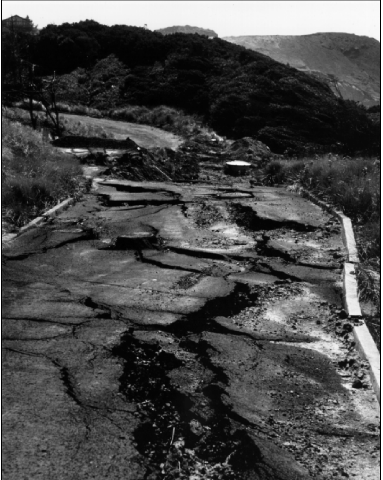
This subdivision along the oceanfront at Newport received a favorable geotechnical report and was approved by the city. Roads and utilities were installed, but the property began sliding seaward before any houses could be constructed. The engineering geologist involved lost his license (P. Komar photo).
