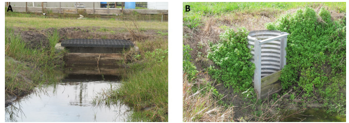
Figure 6. An example of two types of riser-board control structures present on aquaculture facilities in Florida. The image on the left (A) shows a concrete structure with visible riser boards while the image on the right (B) shows a less expensive alternative using galvanized steel pipe.
