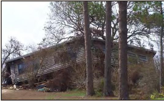
Figure 5-1: A collapsed home on Carabelle Beach (Source: Rosalyn Kilcollins)
