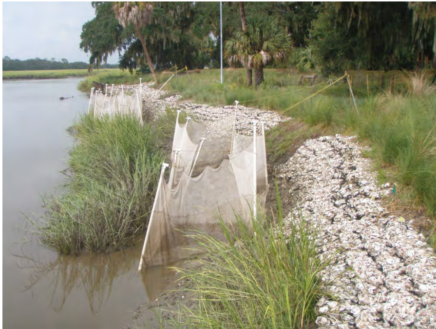
Figure 32. Bottomless lift nets after deployment, at low tide, after construction of the living shoreline.
