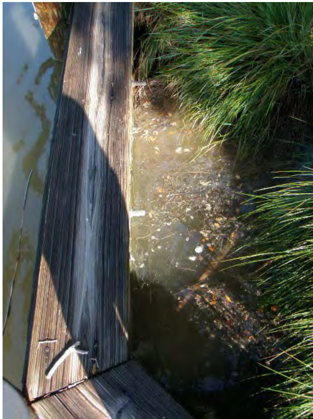
Figure 3. Picture of water infiltration on land side (right of bulkhead) of bulkhead on Little St. Simons Island.
