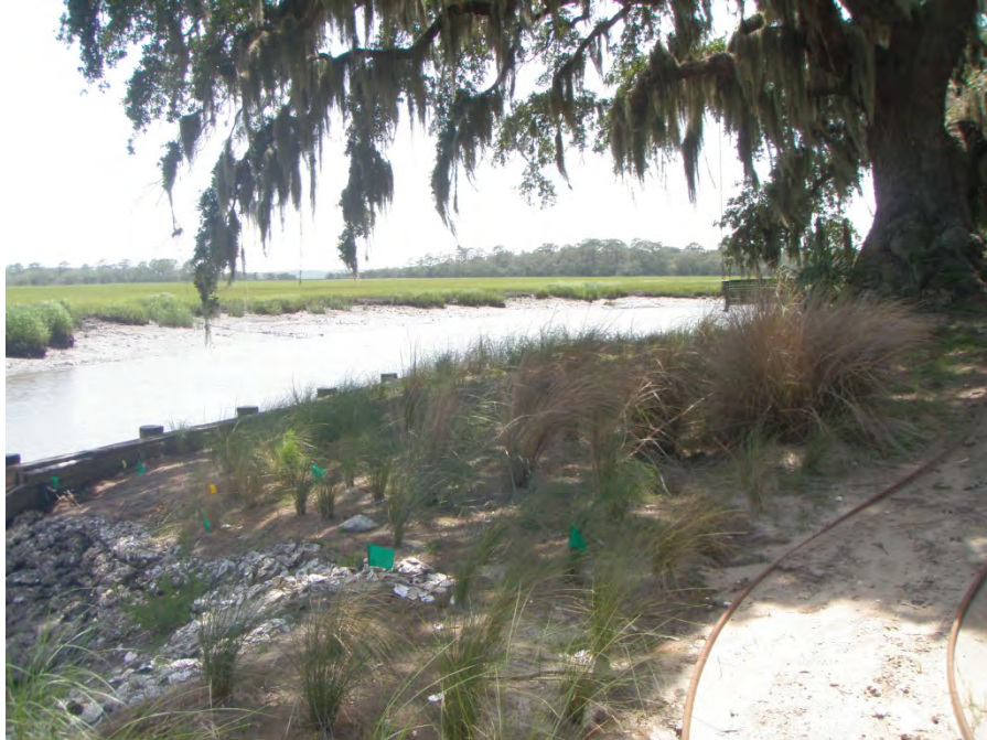
Figure 29. Flagging (dark green) set out in June 2013 to monitor for erosion, Little St. Simons Island, Ga.
