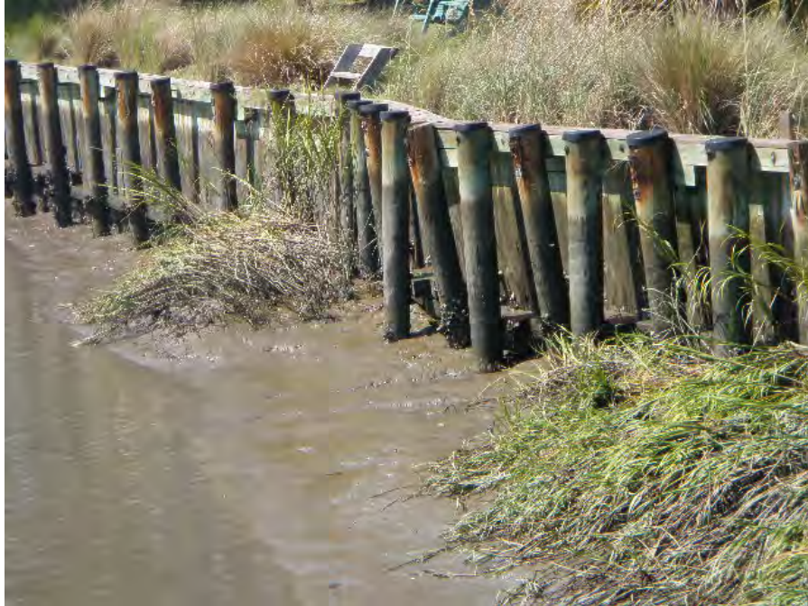
Figure 2. Picture of failing bulkhead on Little St. Simons Island.
