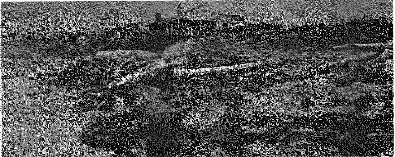
Fig. 10. Same area of the spit as in Fig. 9, showing where waves have washed over the riprap line causing some erosion of the riprap as well as the property.
