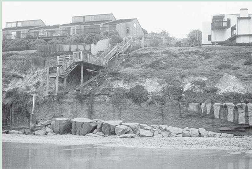
Homes built on actively eroding bluffs in San Diego County are no longer fully supported from below, making them vulnerable to landslides and earthquakes. Photo: California Sea Grant archives
