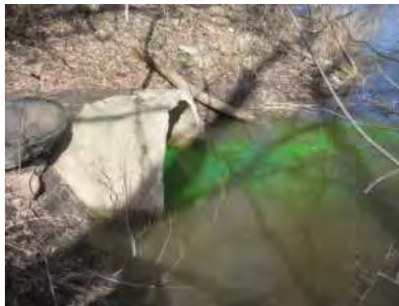
Figure ES-4. Fluorescein dye, which was introduced into sanitary facilities within Miller Park, was released through a stormwater outfall on the Menomonee River.
