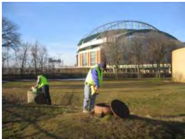
Figure ES-3. Dye testing of sanitary sewer lines near Miller Park. Testing for the human Bacteroides genetic marker was positive in a nearby stormwater outfall.
