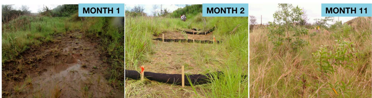
Figure 9 Time series photographs of Restoration Plot 2 Sock Plot (SP). An eroding hillside was chosen for treatment. Sediment filter socks were installed and Acacia auriculiformes tree seedlings were interspersed between the socks. The area was nearly completely revegetated after 11 months.
