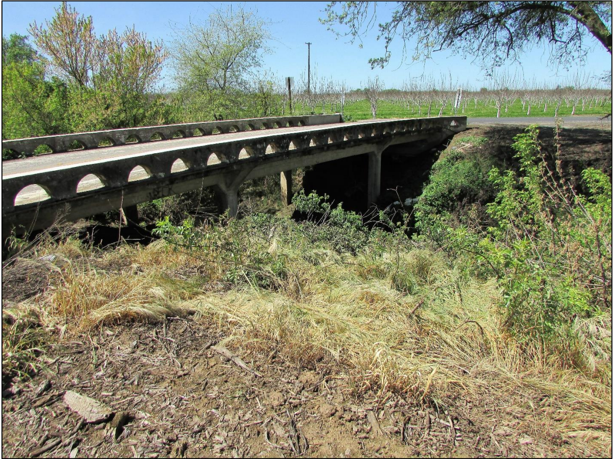
Representative Photo 5: Representative of the Pezzi Road Bridge, taken March 2017; facing north.
