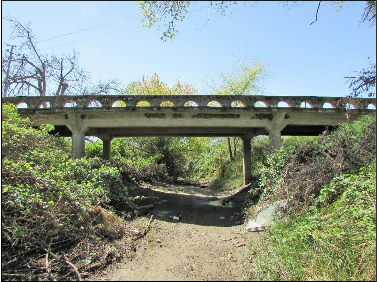
Representative Photo 6: Representative of the Pezzi Road Bridge, taken March 2017; facing west.
