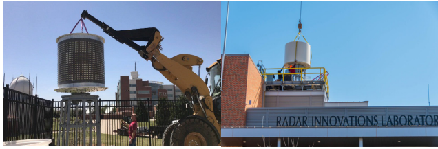
Fig. 1. CPPAR demonstrator. (a) On the ground. (b) Moved to ARRC rooftop.
